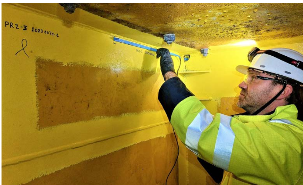
↑ CRATUS crack sensor installed inside a crane girder
