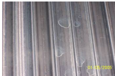
Dry spots and/or white rust
